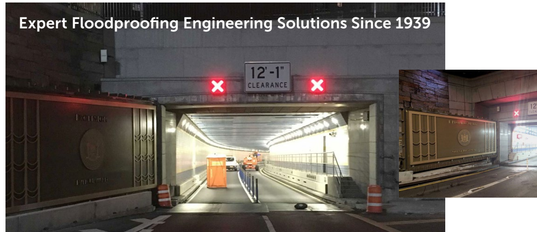
Flood Gates Protecting NYC Queens Midtown & Hugh L. Carey Tunnels From Flooding
